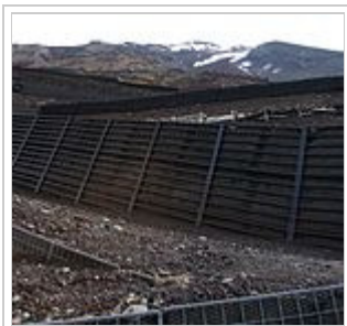
Switchbacks and retaining walls along the trail reduce erosion from the large number of climbers.
